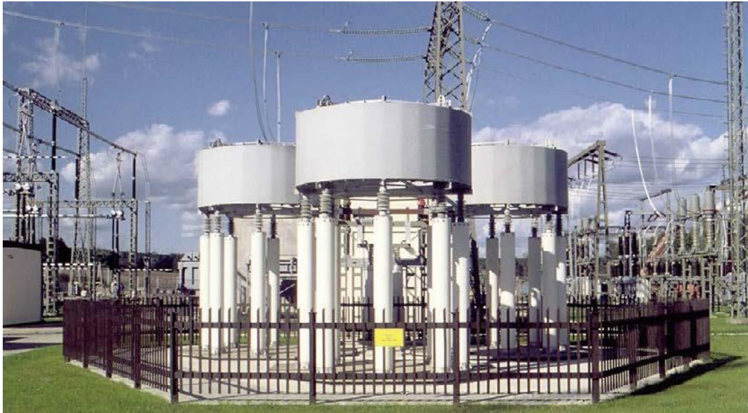
Figura 35 - shunt capacity reactor - fonte Siemens
