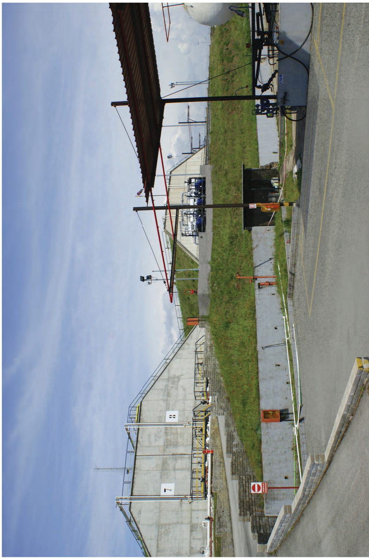
AREA SALA POMPE_POST OPERAM
