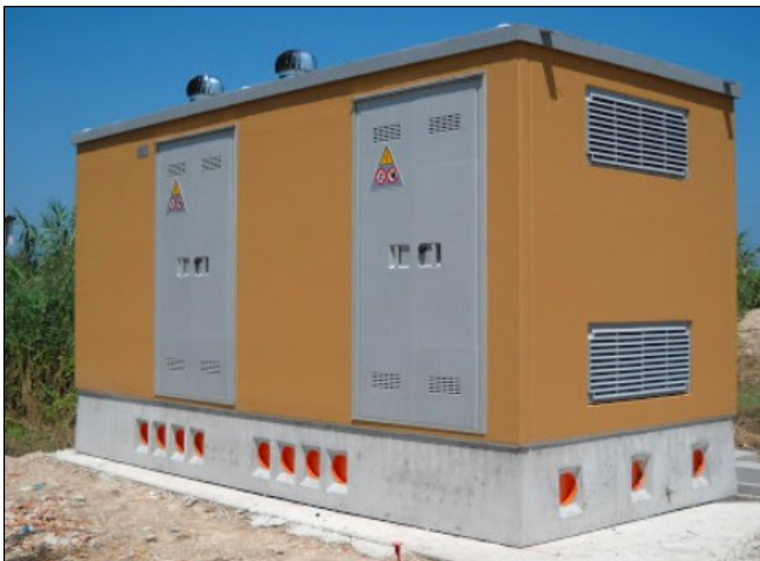
Figura 9 cabina in CAV
