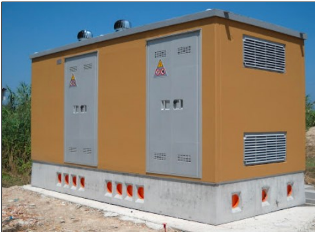
Figura 16 cabina in CAV
