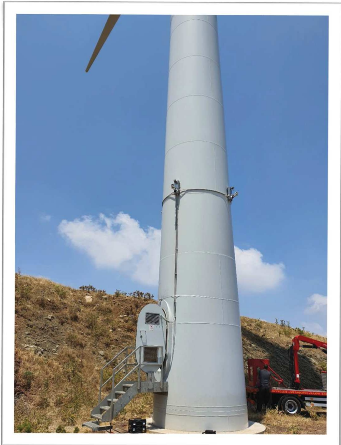
[Outside installation overview – SIEMENS GAMESA]
