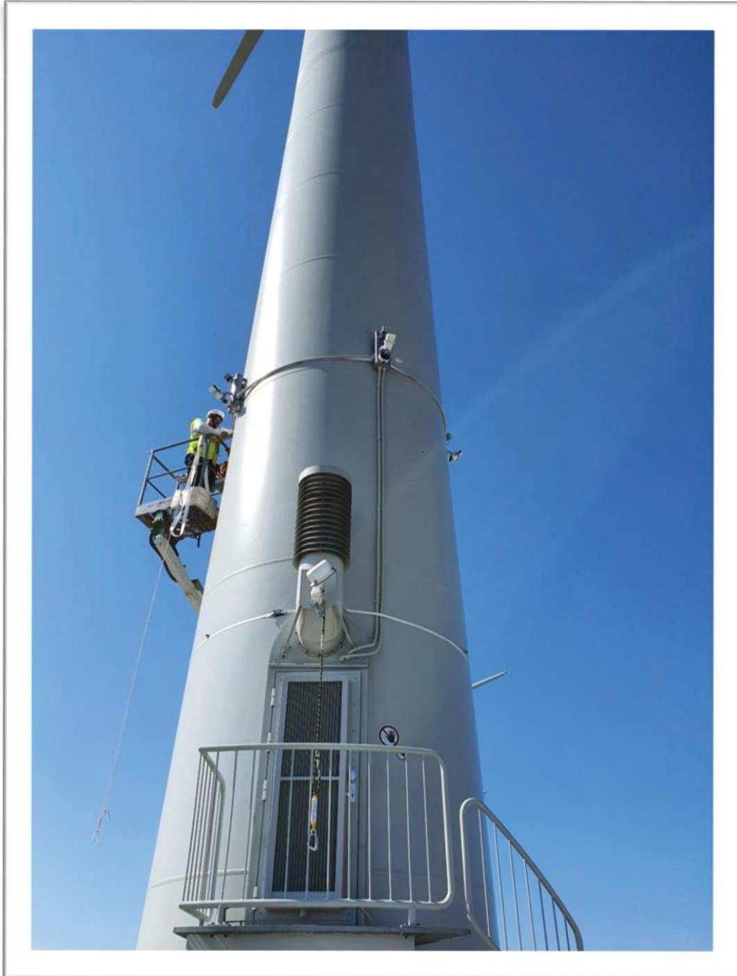
[Outside installation overview – ENERCON E44]
