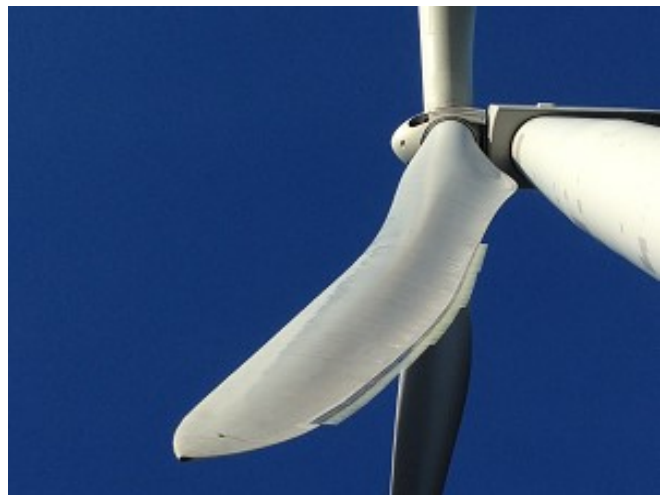
Figure 1: LNTes at the wind turbine rotor blade
