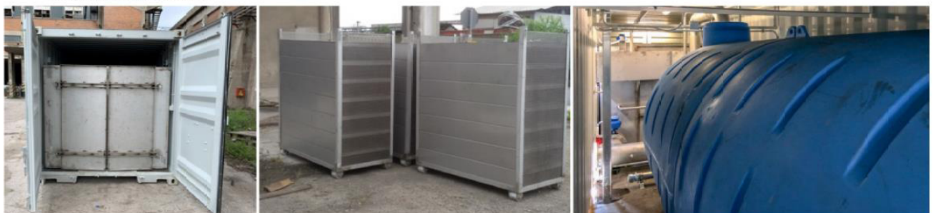
PHOTO OF TREATMENT PLANT
