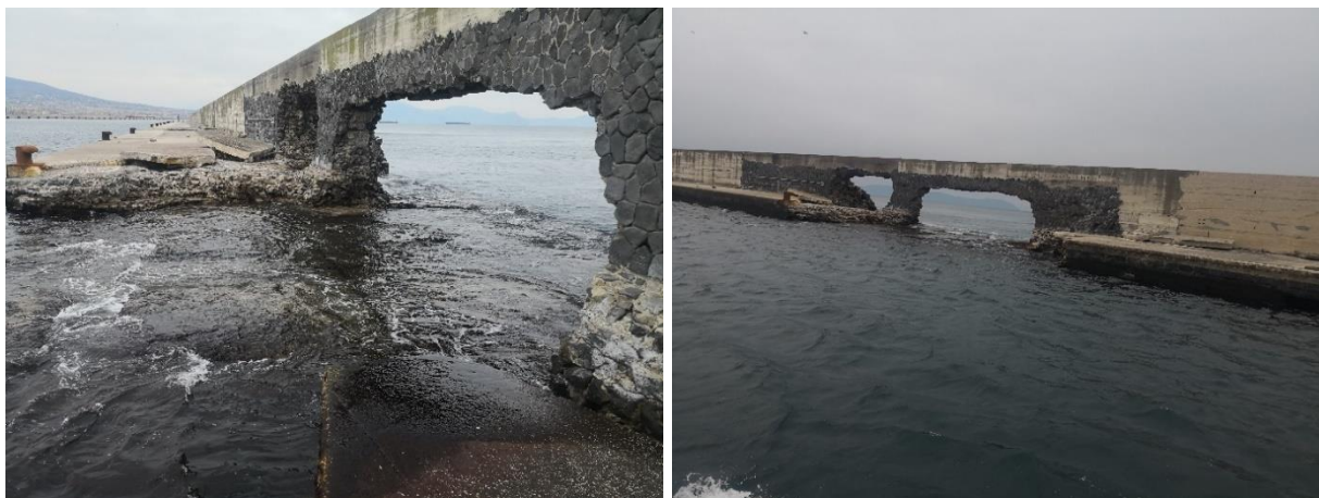
Figura 2 – Dissesto tra le progressive 1+133 – 1+169
