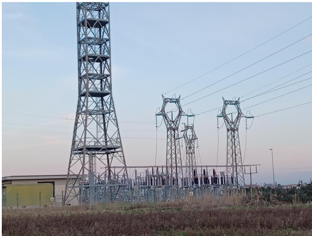
Figura 21 – Cabina Primaria “Caorle” 150/20 kV.
