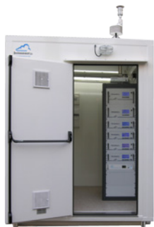
Example of fixed air quality monitoring station with rack version 2M series analyzers.
