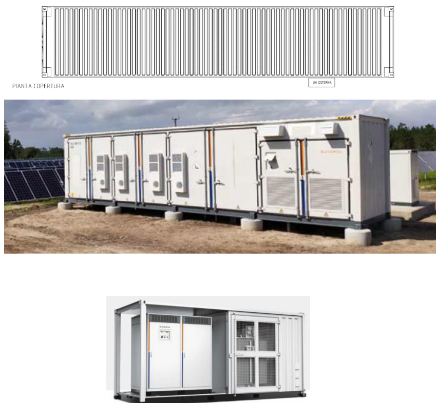
Figura 43 – Container Storage e Power Converter System
