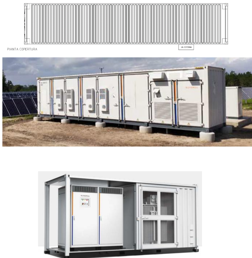
Figura 16 – Container Storage e Power Converter System
