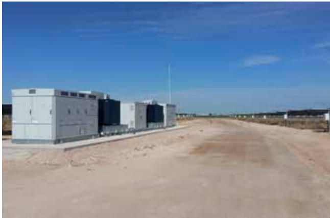
SPAIN Alcázar, 168 MW HEMK+ TWIN SKID
