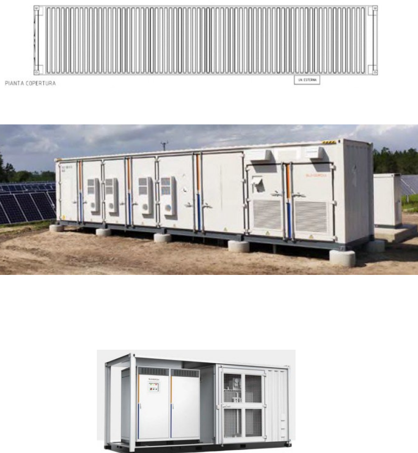
Figura 11 Container Storage e Power Converter System – PCS
