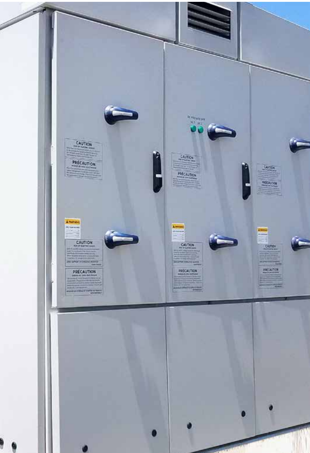
HEM Solar inverter
