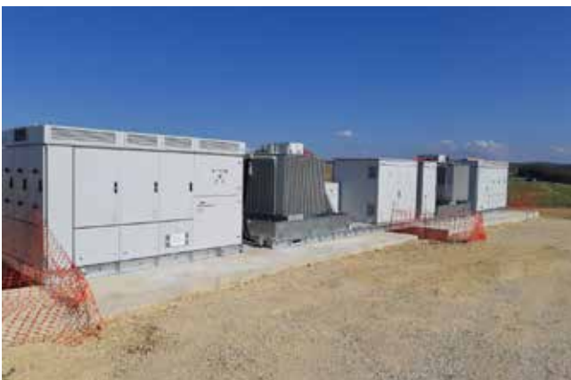
SPAIN Guillena, 105 MW HEMK+ TWIN SKID
