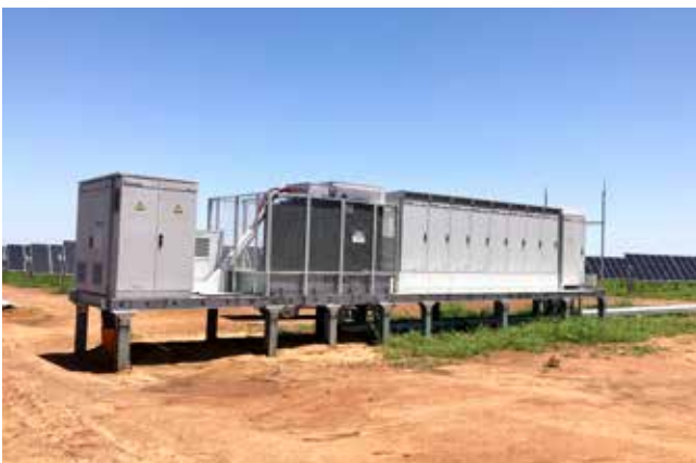
AUSTRALIA Rugby Run, 83 MW HEC V1500 + MV SKID
