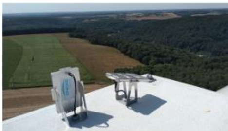
NRG deterrent speakers fixed to nacelle
