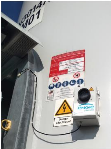
The ultrasonic detector at the turbine base
