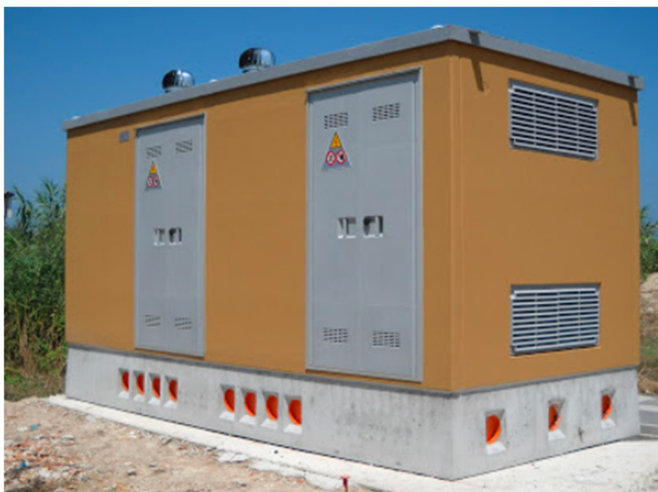
Figura 4 - Cabine in CAV
