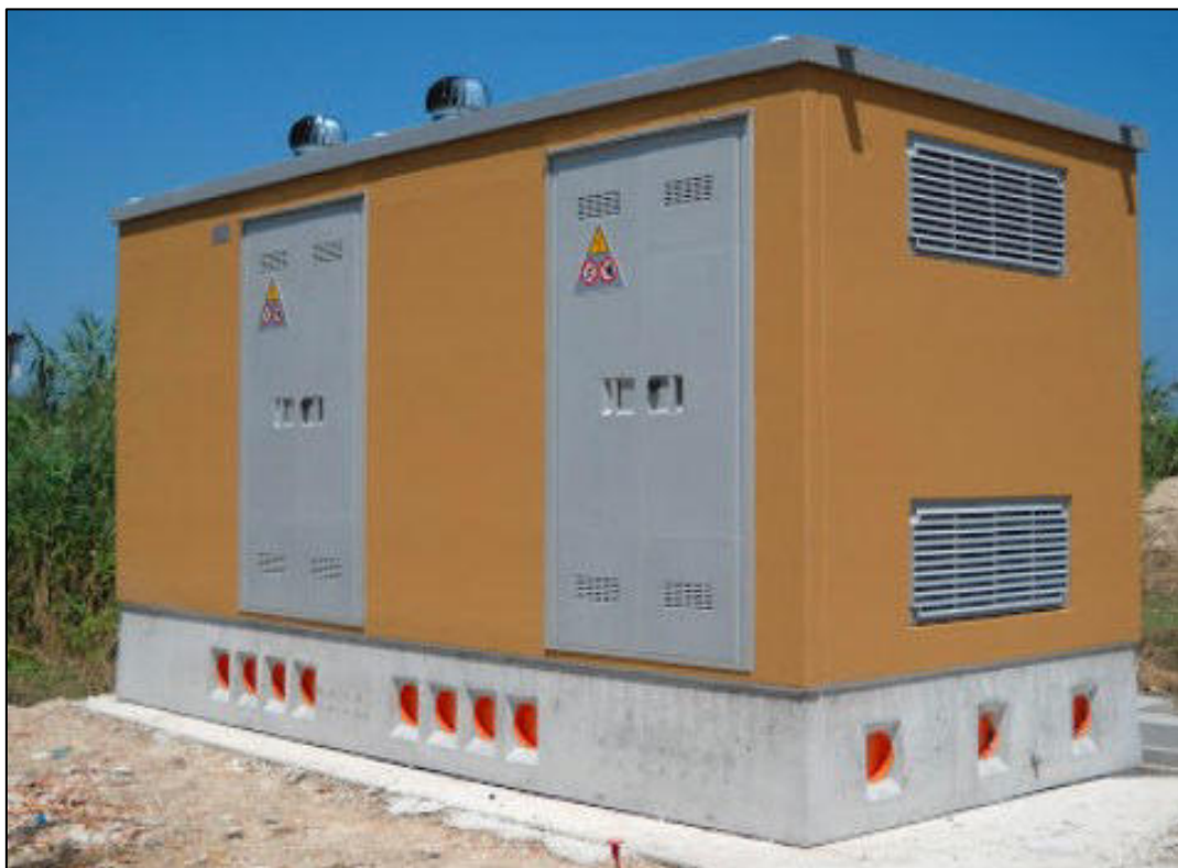
Figura 79 cabina in CAV
