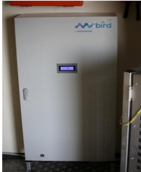
Control unit installed
