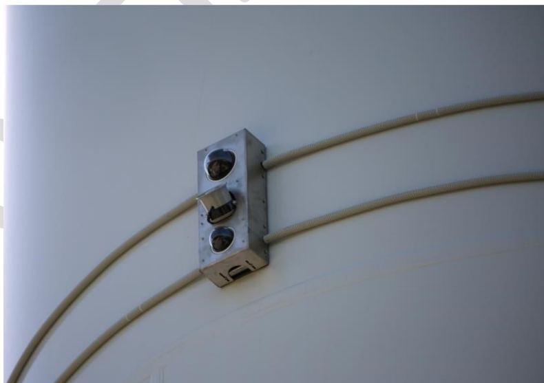
Stainless steel cover with cameras and speaker installed
